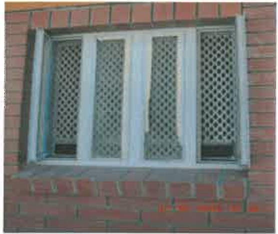
Poor building infrastructure
