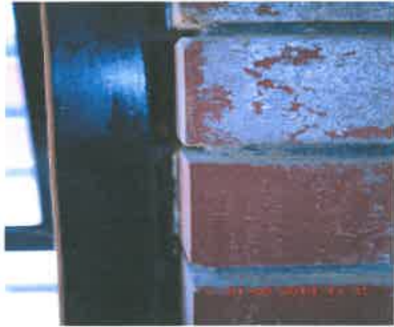
IMAGE 1 & 2: Poor building infrastructure
